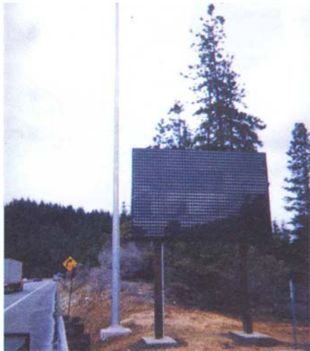
Figure 2: A typical installation. The cameras are mounted on the pole to the left of the DMS
