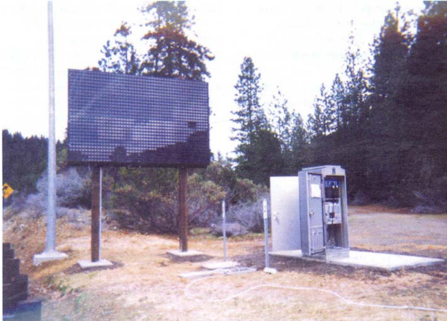
Figure 3: The same installation, showing the location of the control cabinet
