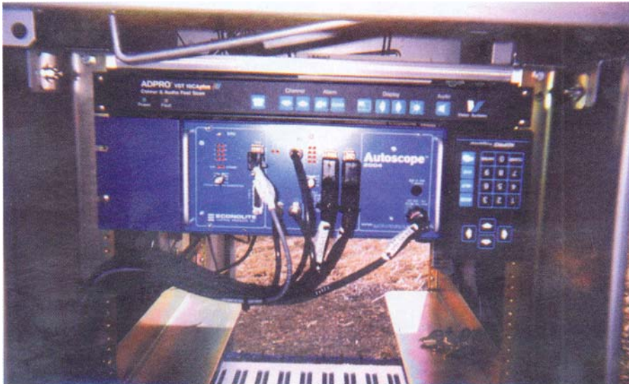
Figure 4: Inside the control cabinet. The Autoscope 2004 is the lower, blue box. The Adpro Fast Scan is the upper black box and keypad
