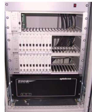
Figure 8: Autoscope RackVision installation at Delnice Control Centre, Croatia
