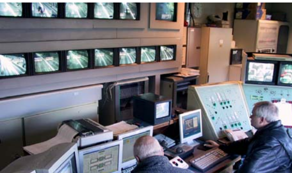
Figure 7: Clyde Tunnel control centre
