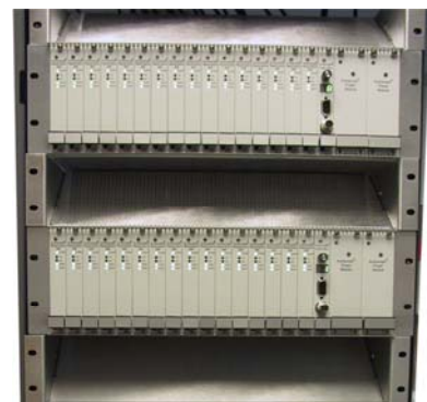
Figure 6: Fully configured RackVision System RVS-16 units to provide 64-camera highway monitoring capability
