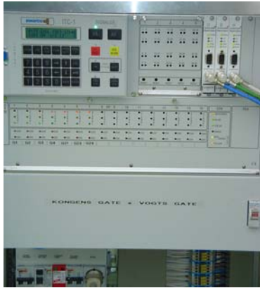
Figure 2: Operational RackVision MVP integrated into the Swarco ITC-1 signal controller for junction control
