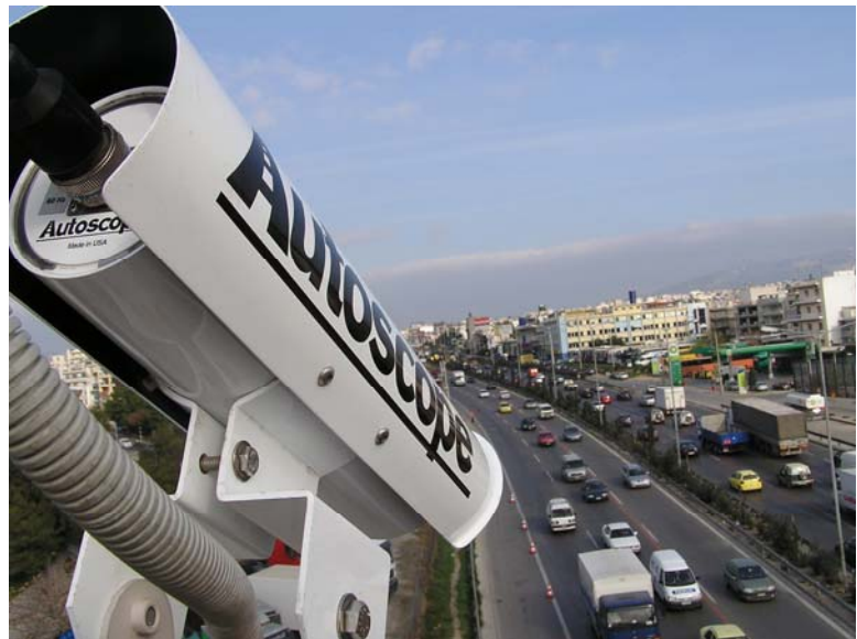
Figure 1: Autoscope camera installation in Athens, Greece
